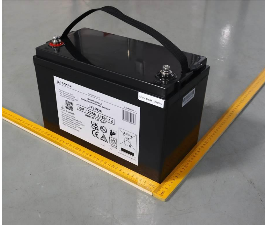
Figure 1 Overall view I of battery
